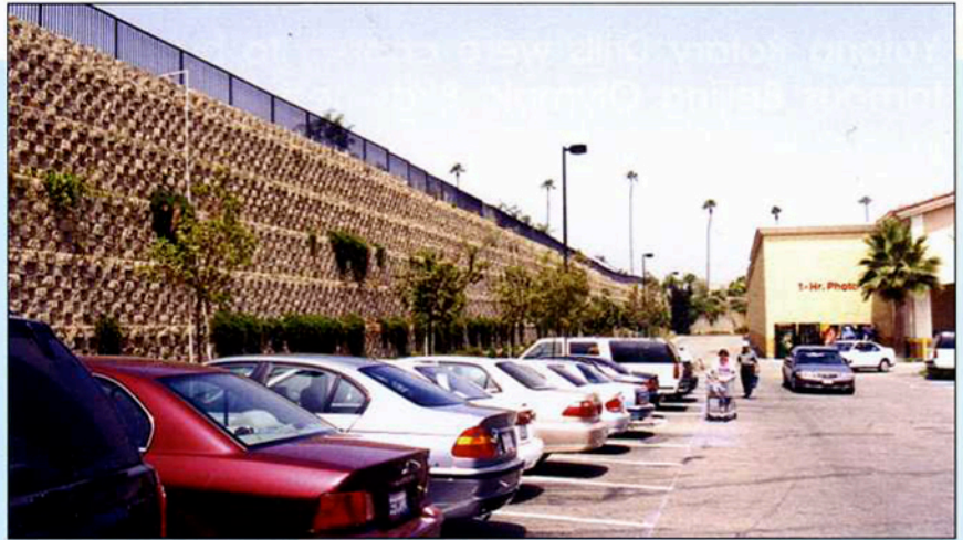
The condition of the "wall" to be replaced prior to new construction.
