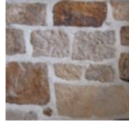
Weathered grout w/ coarse aggregate
